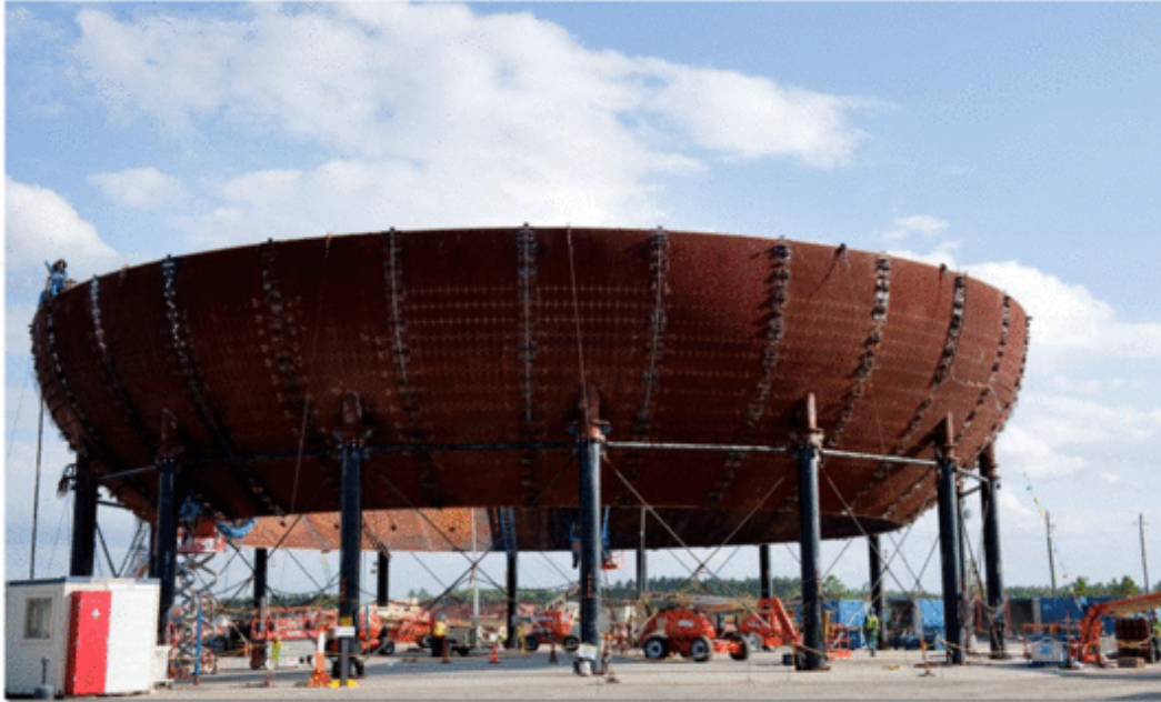
Upper section of Vogtle 3 containment vessel lower head fastened to assembly and welding stand. (November 3, 2011) ©2011 Southern Company, Inc. All rights reserved
